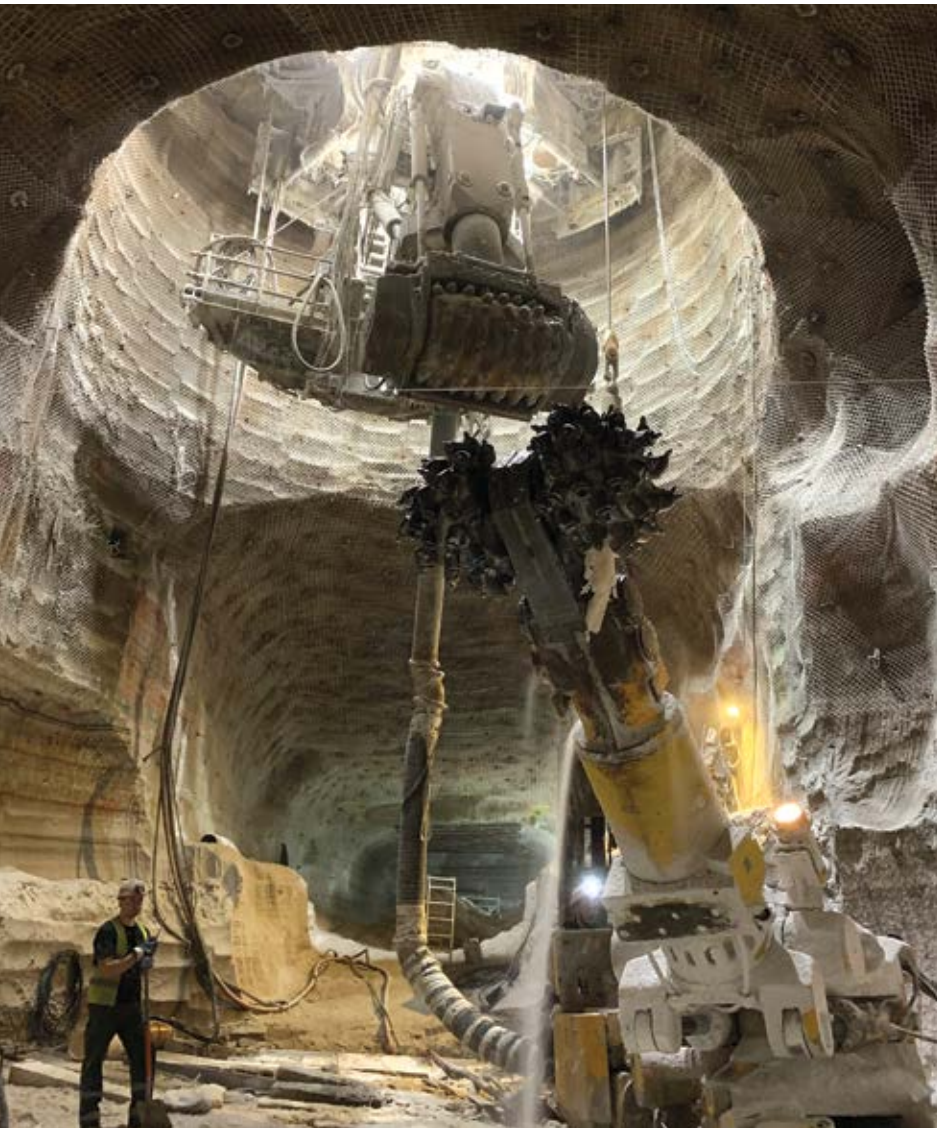
The two shafts at Nezhinsky mine in Belarus are more than 700 m deep and 8 m in diameter. Herrenknecht Shaft Boring Roadheaders do the boring while Redpath manages the project. It is completed fast and with a perfect safety record. (Photo: Redpath Deilmann)
