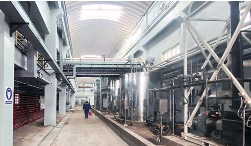
A view inside Shandong Zhongkuang Group’s SART (sulfidization, acidification, recycling and thickening) plant in eastern China. Use of the SART technology at the gold plant, according to BQE Water, allows copper and zinc to be recovered simultaneously from the leach solution as separate high-grade concentrates.
