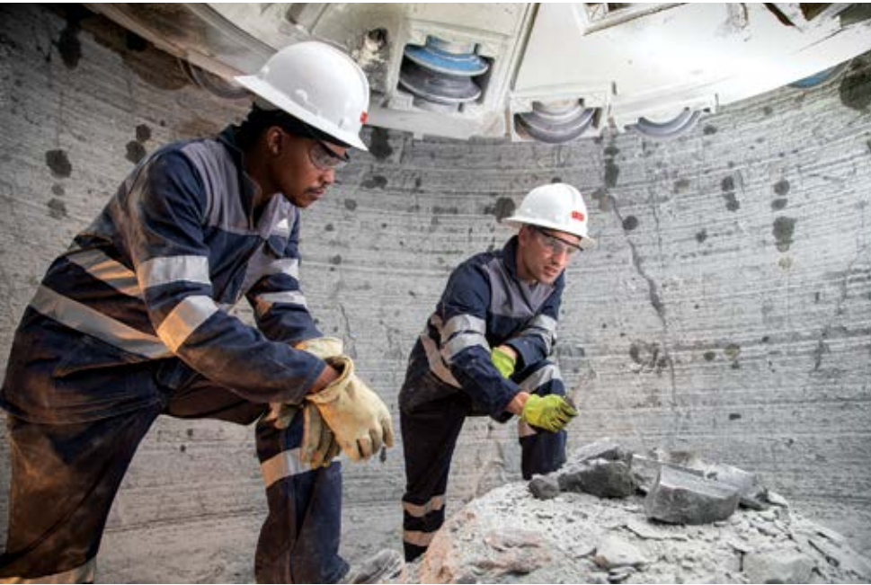
Master Drilling's new Shaft Boring System covers boring, mucking, reinforcing and lining. After a successful field trial, it is recently adopted for a mine in South Africa. (Photo: Master Drilling)
