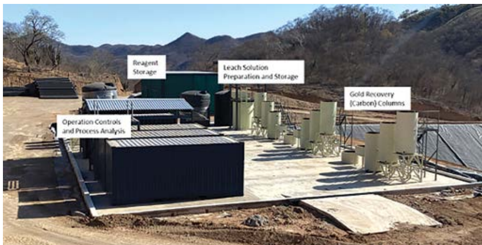
The construction activities related to the gold recovery plant (above) are now complete.
