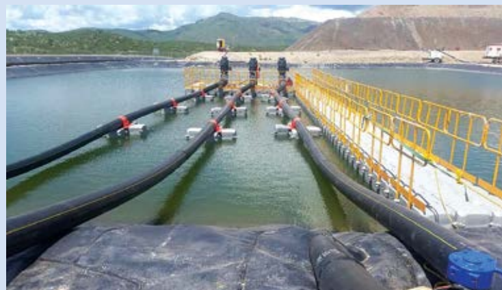
Three Goulds Water Technology turbine pumps on a Xylem custom-built raft unit are a key part of the process water solution. These turbine pumps feed high pressure pumps that irrigate the extracted mineral ore.
