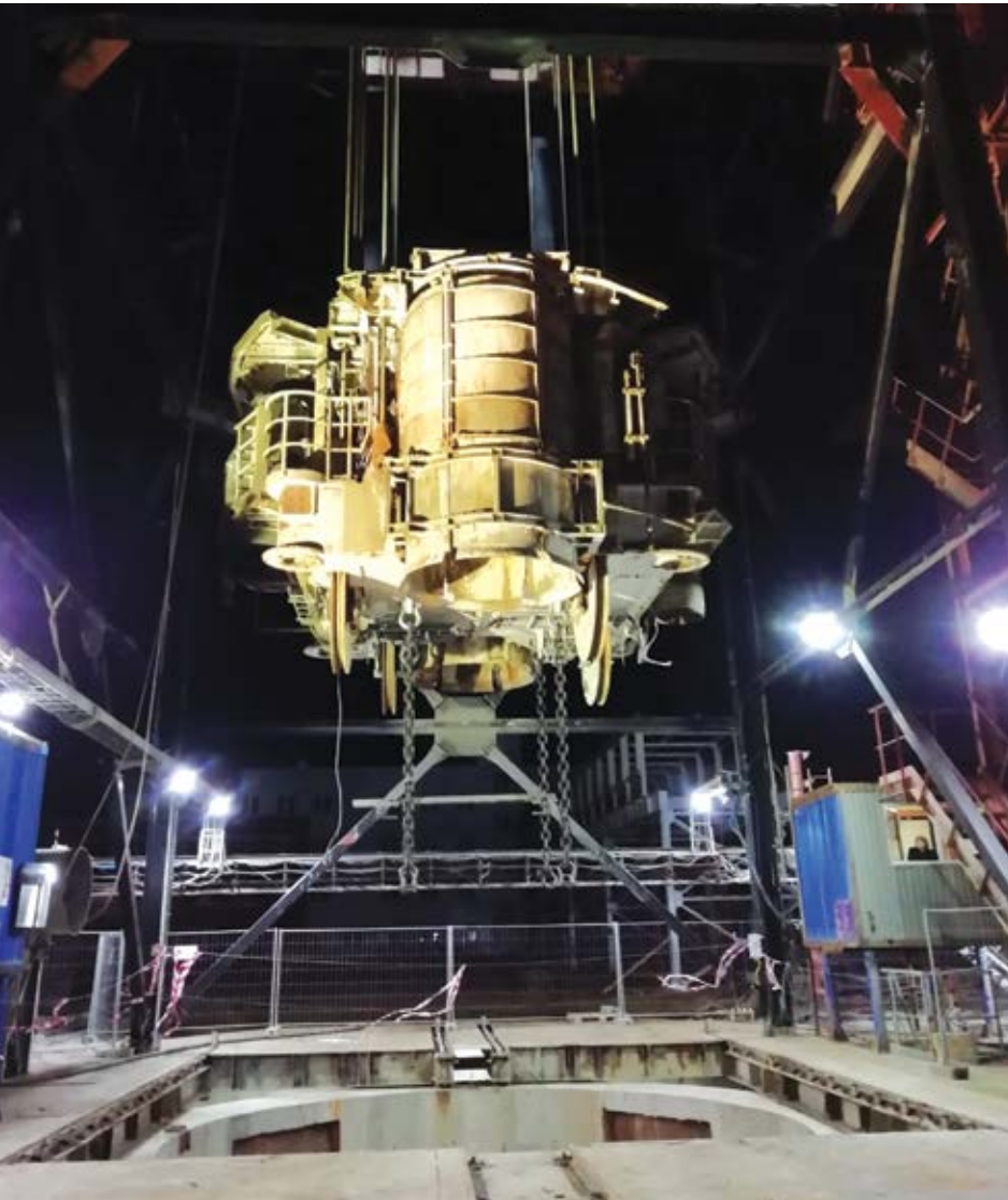
On October 2020, the last Herrenknecht SBR is hoisted out of Shaft 1. (Photo: Redpath Deilmann)
