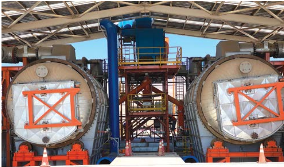
The thermal conversion reactors at Kal Tire's OTR tire recycling facility in Antofagasta, Chile, uses heat and friction to help reduce tires to their component elements. (Photo: Kal Tire)
