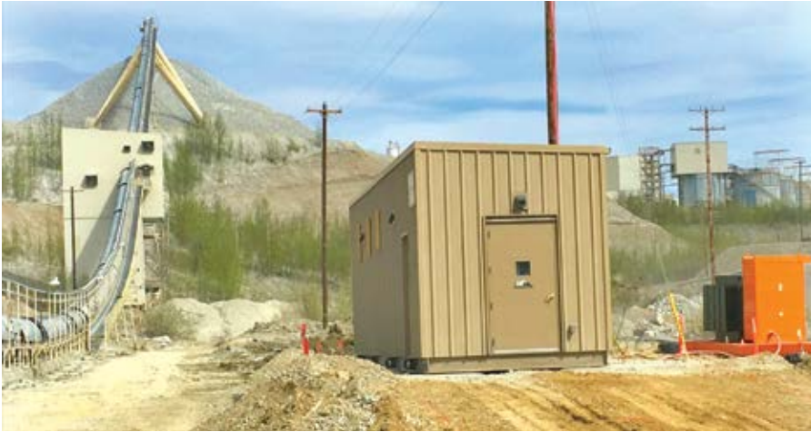
Ehouses offer an economical, easily relocatable and flexible solution for mines that need to house and protect pump controls and other low- to medium-voltage equipment in remote areas. (Photo: Morrison-Maierle)
