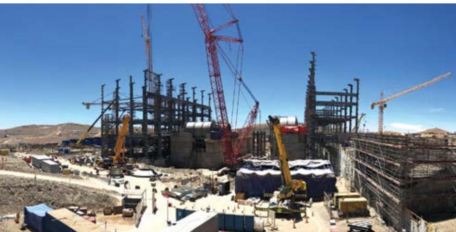
Construction activities resume, such as the trunnions for the grinding line at the QB2 project (above).
