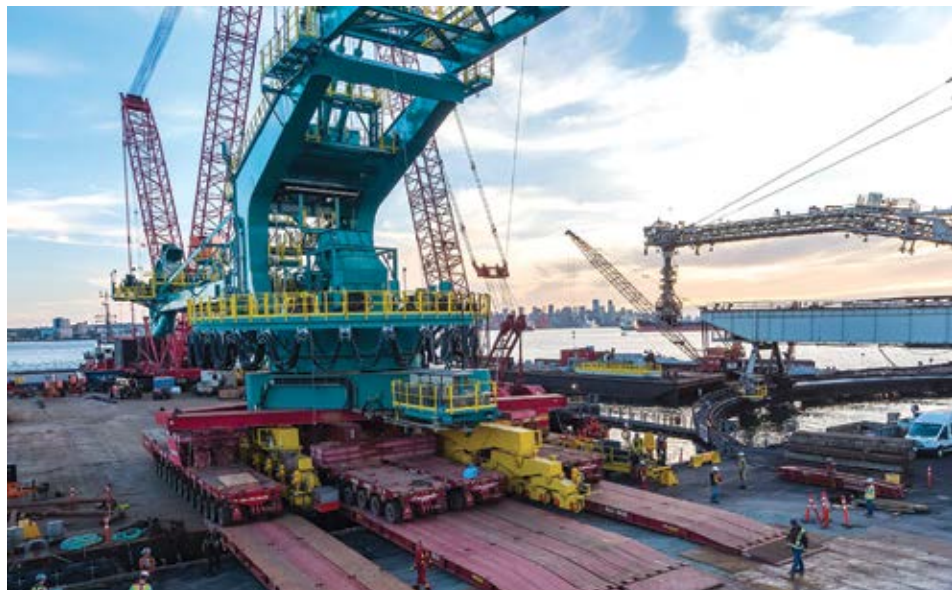
A 79-m-long stacker is offloaded by 66 axles of Self-Propelled Modular Transporters at Neptune Bulk Terminals in Vancouver, Canada. (Photo: Mammoet)
