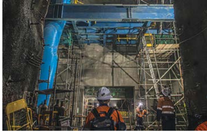
The conveyor decline at Oyu Tolgoi continues to progress with 900 m completed during the last quarter.
