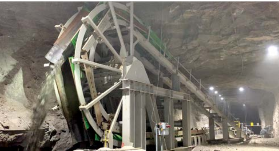
The standard Rail-Veyor car is 2.4 m long. Recently, the company designs a 1.5-m car for a smaller discharge loop. (Photo: Rail-Veyor)
