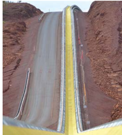
The 14-km overland conveyor for BHP’s South Flank operation in the Pilbara incorporates horizontal curves for increased power and efficiency, and lower capex and opex. (Photo: Fluor)
