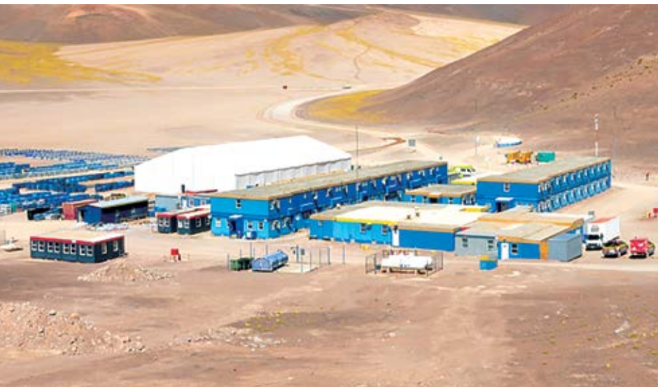
About 15% of the total construction has been completed to date, including the 1,800-person mining camp (above).
