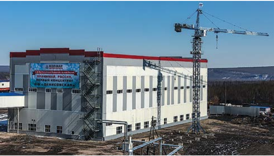
Kolmar starts construction of the second stage of the Inaglinskaya coal complex.
