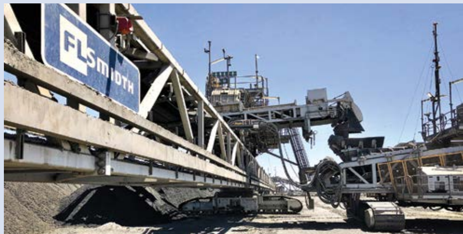
In addition to dry-stack tailings, FLSmidth has identified other opportunities to reduce waste and emissions.
