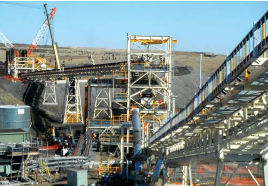
Construction of the parallel coal handling facility at Glencore's open-cast Rolleston mine. WSP designs the plant on time and within budget. (Photo: WSP)
