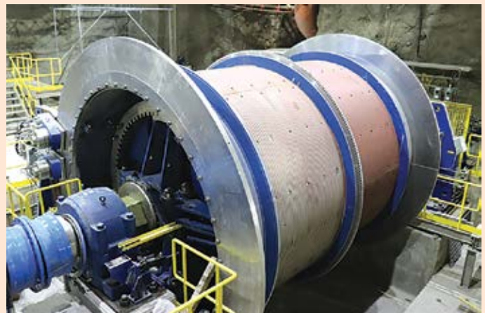
The internal hoist at the bottom of the Craig mine will eventually lower miners to the 2,630 level.
