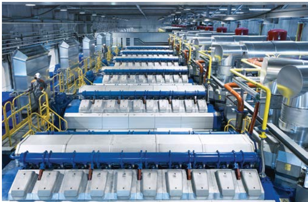
The fast-starting Wärtsilä 34DF generating sets that will power Grasberg’s underground mining operations can run on biodiesel and natural gas. (Photo: Wärtsilä)
