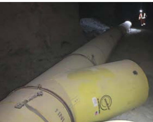
At a salt mine in New York, Turnstone Industrial Solutions installs 30-in. HardLine-MAX ducting. It conducted 15,000 cfm to the face and led to a ‘big win’ contract for a turnkey package. (Photo: Turnstone Industrial Solutions)
