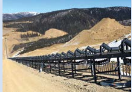
A Yukon gold mine recently installs this overland conveyor with PPI structure and hardware.
