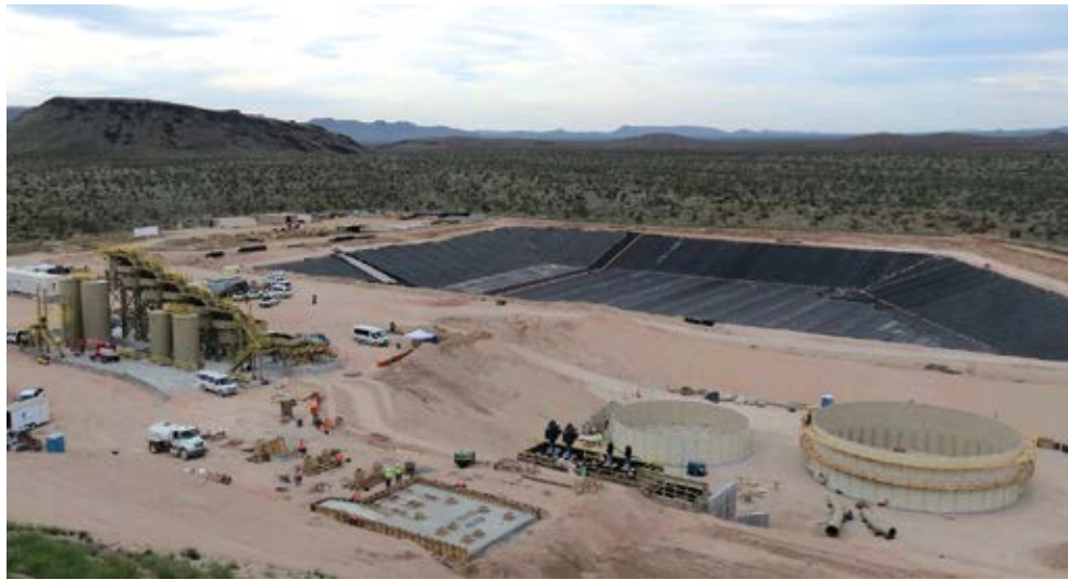
New barren and pregnant solution tanks sit in a containment area (foreground), while construction is completed on the carbon-in-leach plant (left).
