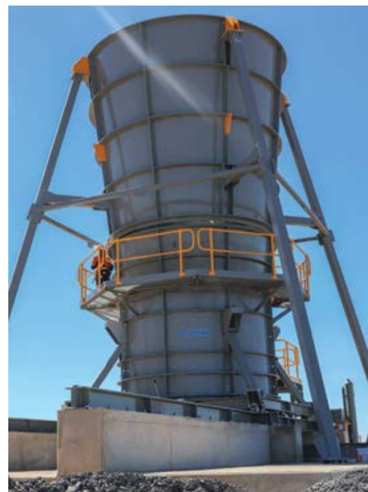
In 2015, Zitrón S.A. installs the massive 5,600-kW ZVnV 1-36-1400/8 fan system at the Dugald River mine in Queensland, Australia. (Photo: Zitrón S.A.)
