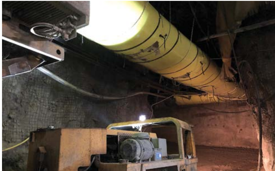
A gold mine in Washington state contracts Turnstone for more than 1,000 ft of 60-in. oval HardLine ducting. The HDPE-based polymer tubing maximizes airflow for the space available. (Photo: Turnstone)
