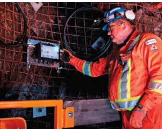
Plexus PowerNet delivers high-speed connectivity to the face at MacLean's test mine in Sudbury, Canada. (Photo: MacLean Engineering)
