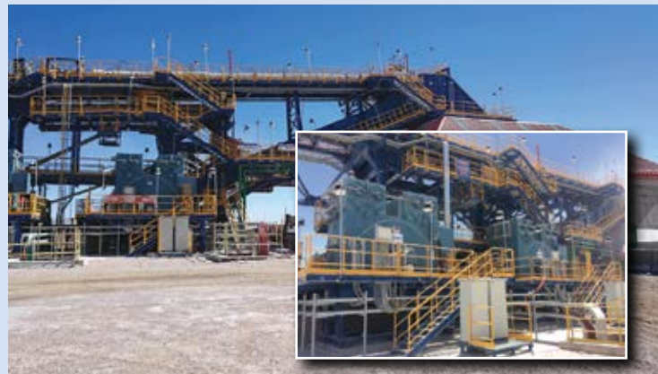
The overland conveyor’s discharge at the mineral processing facility employs four 5-MW gearless drives (inset).
