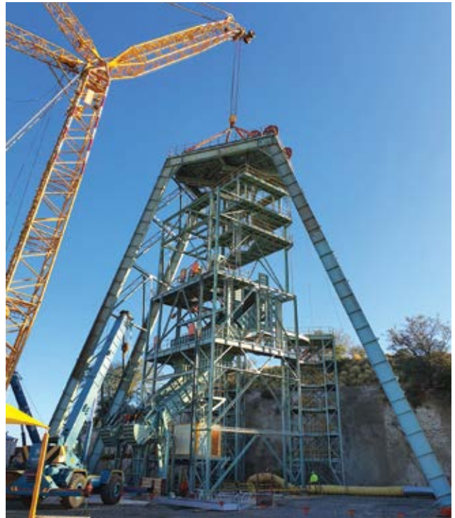
Above, a crawler crane lowers the headgear assembly during the pre-sink phase for a ventilation shaft at Palabora Copper. M&RC reports the pre-sink phase is now complete. The shaft is expected to be completed in Q3 2022. (Photo: M&RC)
