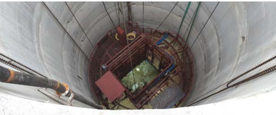
Above, during the pre-sink phase for a 1,200-m-deep ventilation shaft at Palabora Copper, in South Africa, water incursions occurred down to the 50-m level. To answer, Murray & Roberts Cementation use a quick-setting chemical compound, concrete lined the barrel, and resealed behind the lining. (Photo: M&RC)
