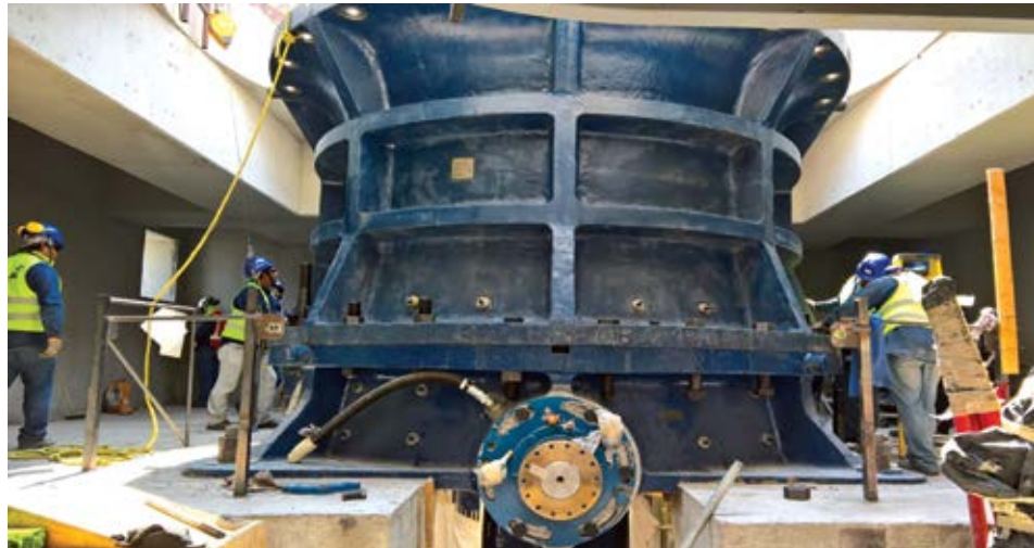
Beneath the surface, maintenance crews work to plan to ensure maximum efficiency and minimal downtime. (Photo: FLSmidth)
