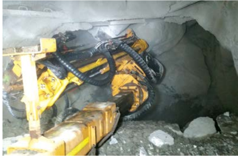
Above, the Auto Explosive Loader drilling a rock and pushing wireless explosives into the hole. (Photo: MacLean Engineering)
