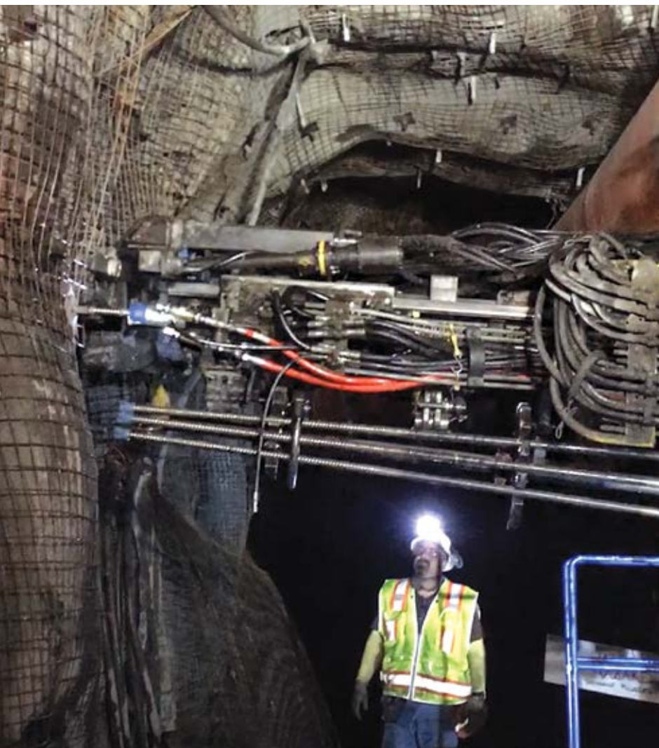
Some American miners working on the Carlin Trend are installing the Nevada Bolt, slang for Jennmar's MPA and J-LOK P resin pumping system (above).
