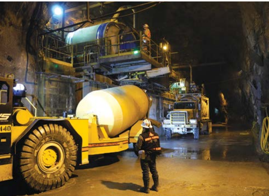
Maintaining consistent quality of large volumes of batched concrete underground is possible and, once they get into a working routine, miners usually find that using shotcrete is extremely versatile, flexible and fast.
