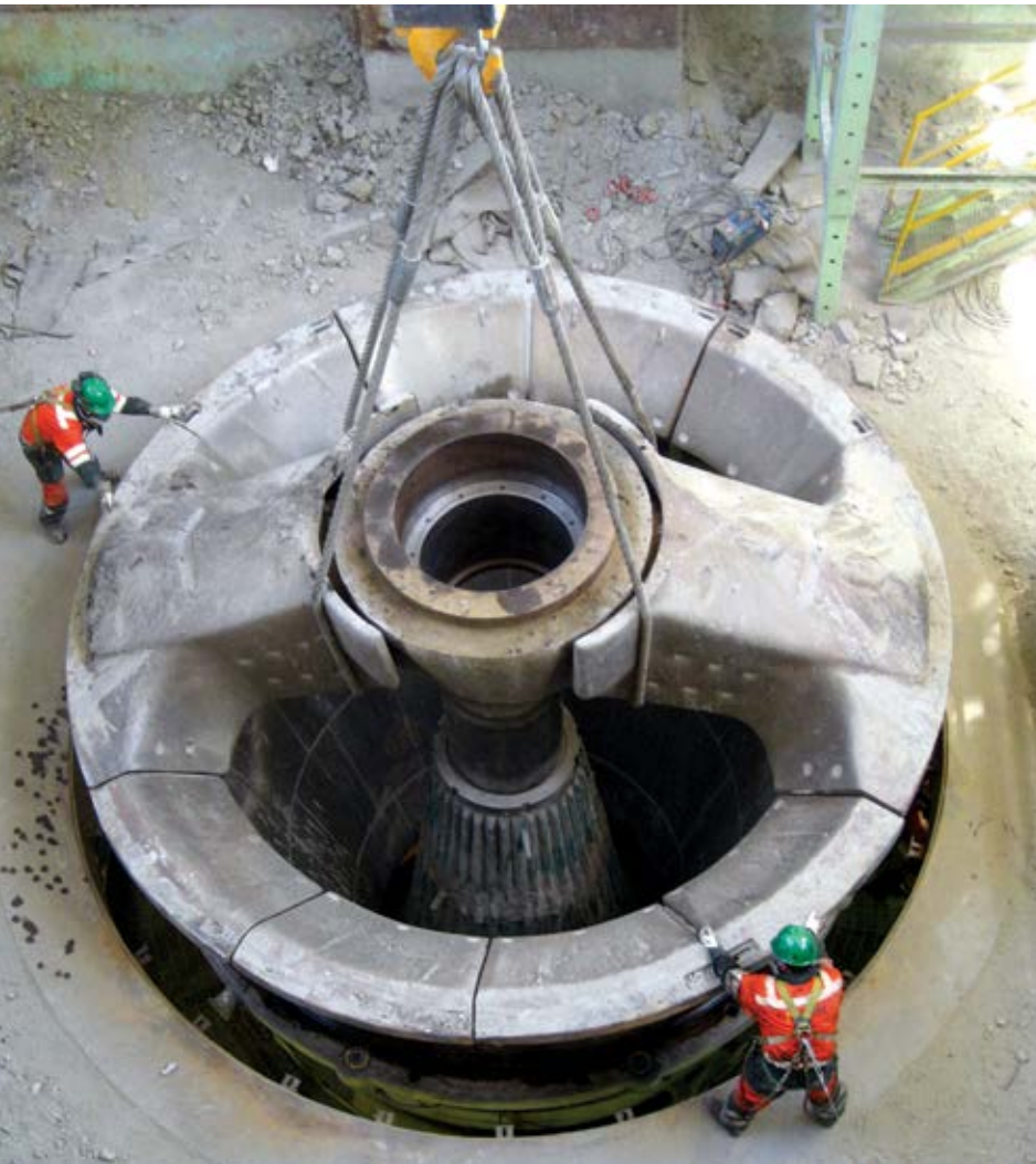
Safety is paramount when working on such large, heavy pieces of equipment. (Photo: Metso Outotec)
