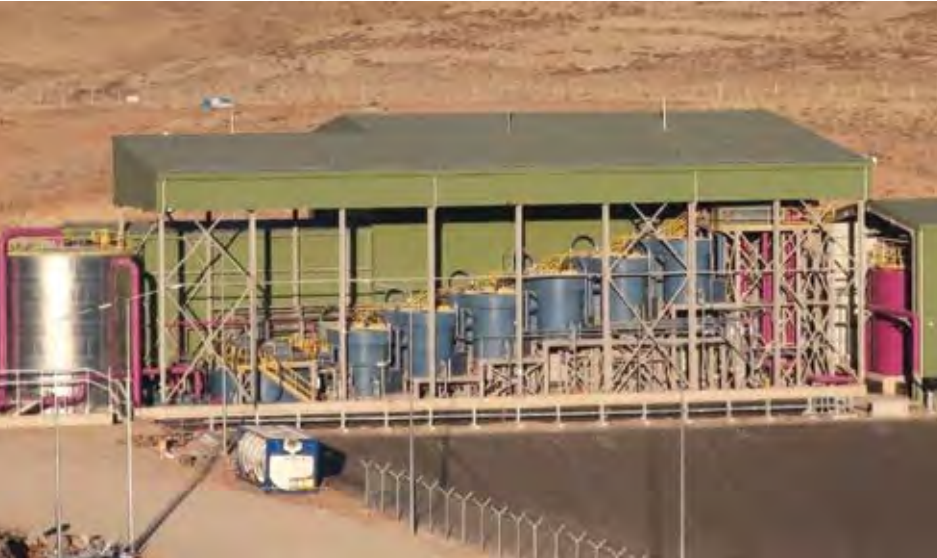
The CIC tanks at Öksüt's ADR plant remove gold from cyanide solution. (Photo: Centerra Gold)
