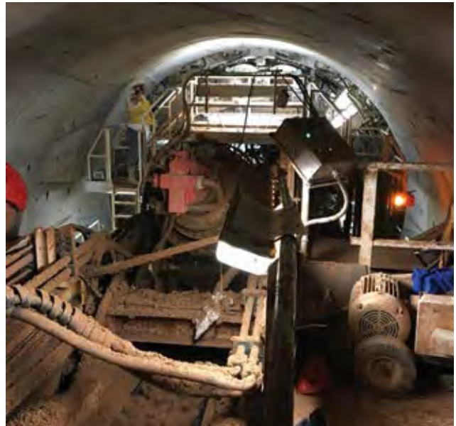
MAPEI's UTT products were used to help a tunnel boring machine dig the Anacostia River Tunnel, which extends for 2.37 miles from Robert F. Kennedy Stadium in northeast Washington, D.C., to Poplar Point in southeast D.C.
