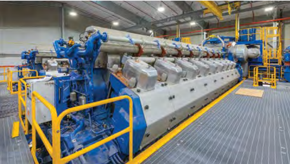
On-site power solutions can include diesel generation technologies, like the reciprocating engine pictured, as well as cleaner or renewable sources of power. (Photo: Burns & McDonnell)
