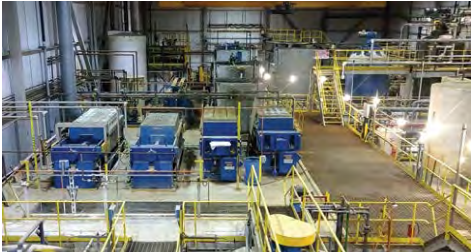
First Cobalt plans to expand an existing cobalt refinery's capacity from 12 metric tons per day throughput to 55 mt/d. Plant feed will come from Glencore's operations in the Democratic Republic of Congo, where cobalt is obtained as a byproduct of copper mining.
