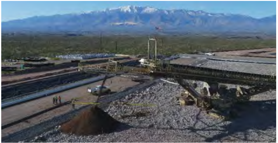
Freeport's Lone Star operation in Arizona begins stacking copper ore on the leach pad.
