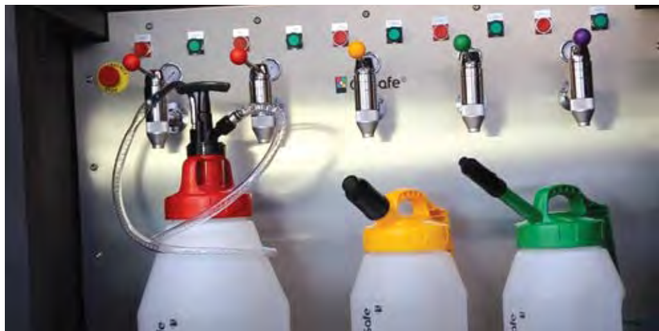
Appropriate lubrication storage equipment and clear labeling of products, through tags, signage or color coding, can reduce the possibility of human error in handling and application.
