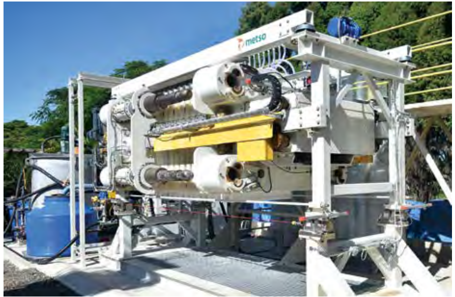
Metso recently installs a VPX 10 filter at its facility in Sorocaba in Brazil to test the technology on different types of tailings and help customers to build a business case prior to purchase.
