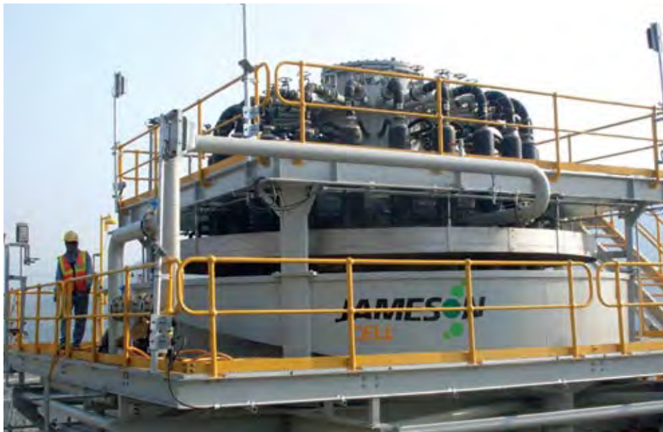
In a move Hudbay reports was based on ‘real-world’ decisions, New Britannia will build a flotation circuit of Jameson cells to handle a feed of widely varying grade fines. (Photo: Glencore Technology)
