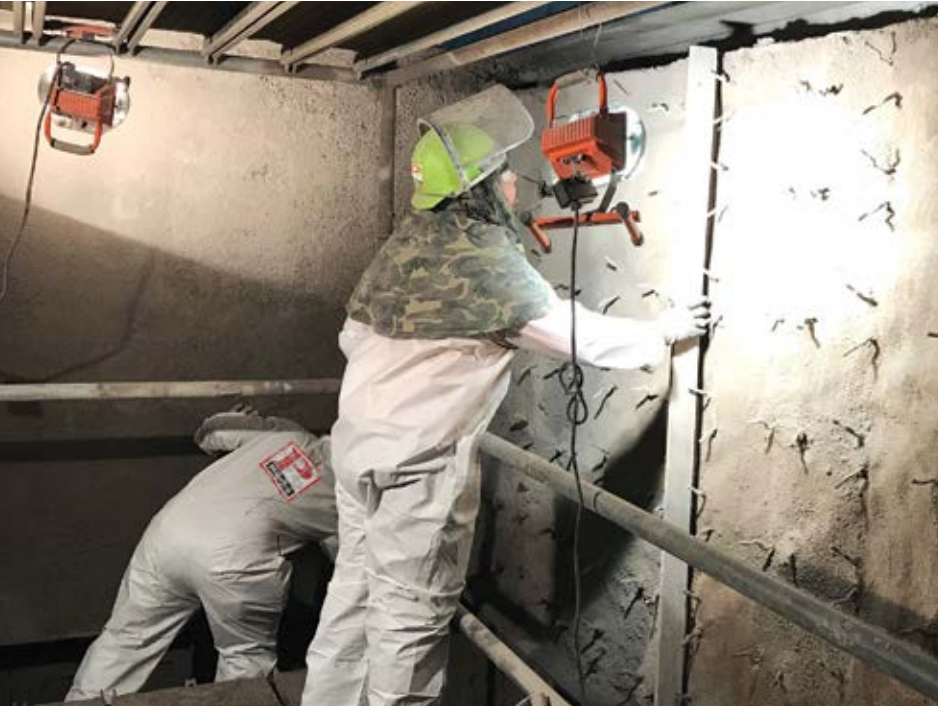
Following industry-standard recommendations for refractory anchor installation can increase service life and maximize refractory performance.
