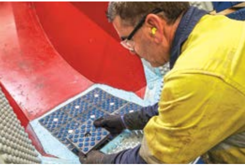
A technician installs FerroCer wear panels. Each panel has a set of abrasion-resistant ceramic inserts enclosed in a matrix of malleable steel.
