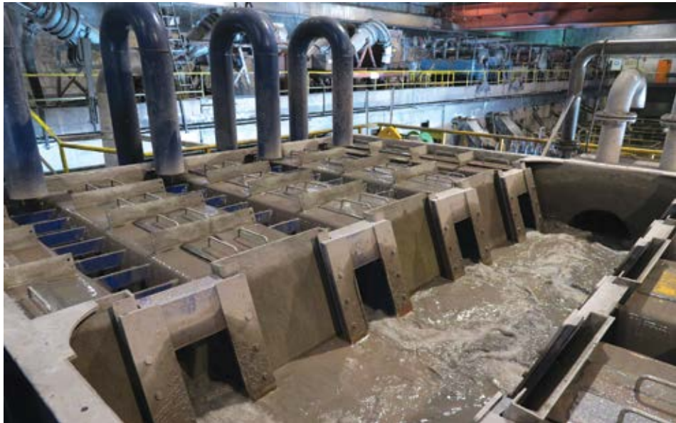
One application for the Reflux Classifier is in the recovery of minerals from tailings as shown in this image of an RC3000 applied to recover high-grade ultrafine iron ore. (Photo: Kevin Galvin)
