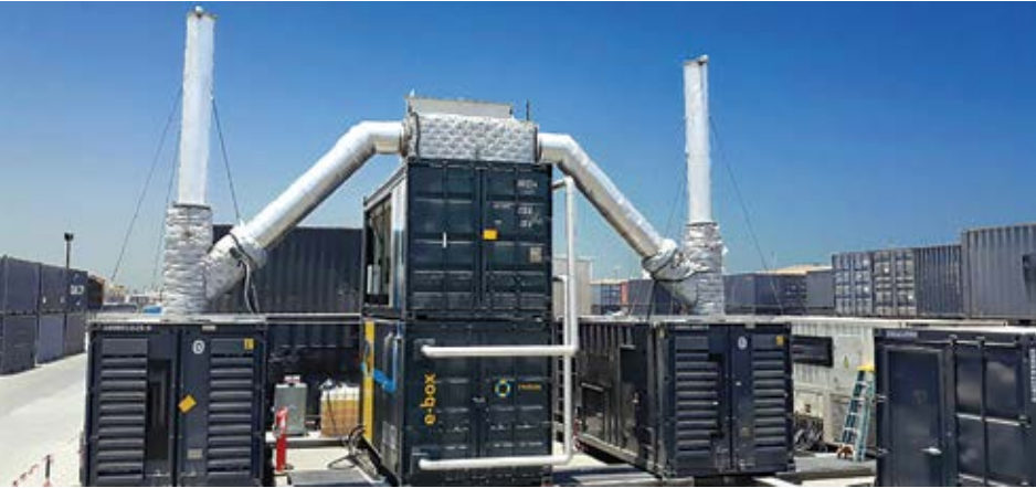
The newest waste heat recovery systems for diesel genset installations are based on conventional steam turbine technology, but at a smaller scale suitable for remote minesite applications.
