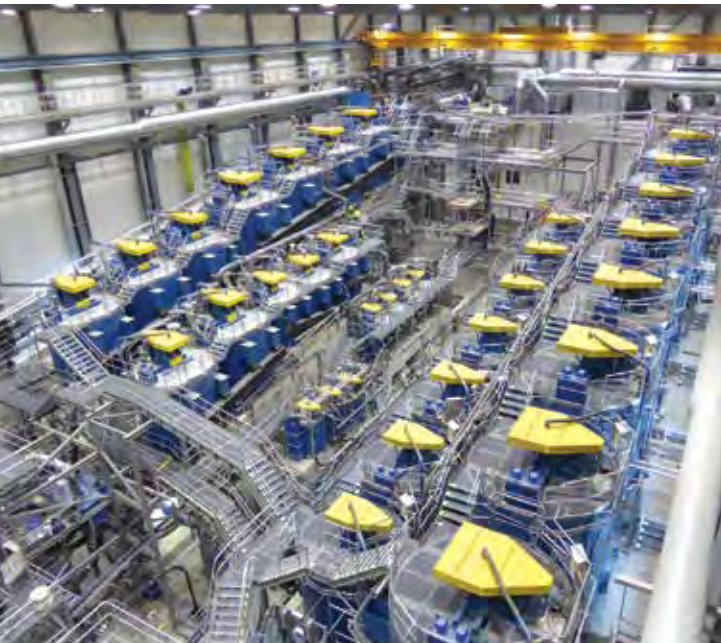
Flotation cells installed at Boliden's Garpenberg zinc mine in Sweden. (Image: Metso)
