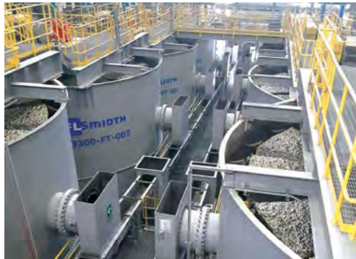
FLSmidth's new mixedROW concept uses a combination of flotation technologies in a clever arrangement to lower energy consumption and improve recovery. (Image: FLSmidth)
